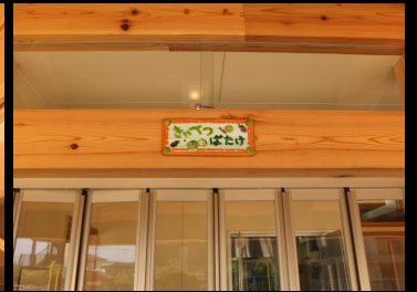
同左室名板＋欄間の通風窓
